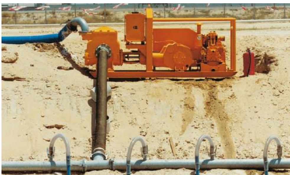
Figure 2. Well points connected with quick release couplings to a ring main header pipeline and pump
